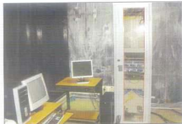
IT Infrastructure at CMC
